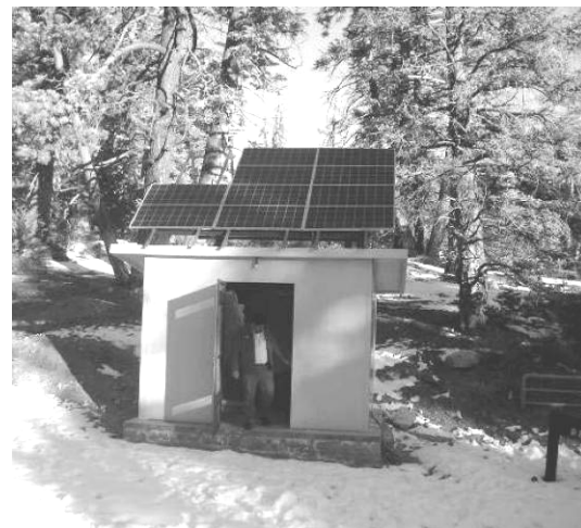
Fig 6. 800 Watt photovoltaic test system with battery and control building (February 2008)
