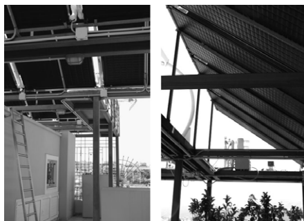
Fig 6. Building's Solar Collectors/Field
