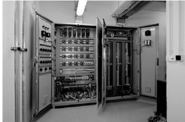
Fig 8. The BMS (Basement)
