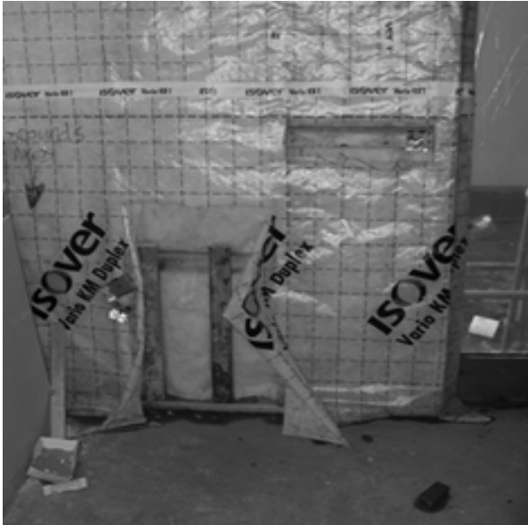
Fig 3. Phase 1 Newcastle, Problems with Airtight Membrane
