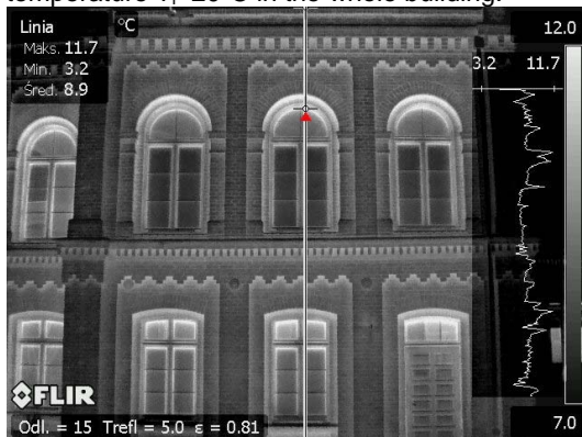
Fig. 9. Results from infrared camera – vertical temperature profile along the elevation.
