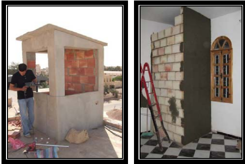
Fig 4: The construction of the wind tower Water was provided directly from the tank. The water was provided from an existing tap on the exterior that could be easily controllable.
