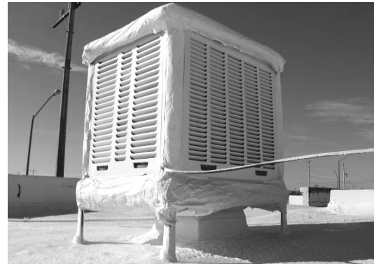
Figure 5 Evaporative cooling system insulated with fiberglass and reflective foil.
