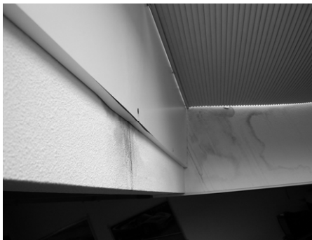
Fig 5. Leakage from roof
