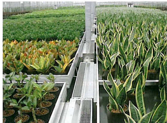
Fig 1. New heating and cooling system in a closed horticulture greenhouse
