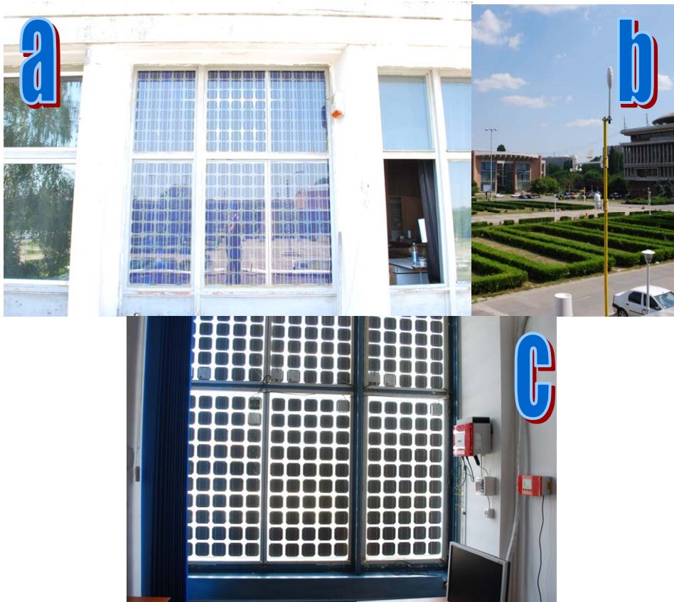
Fig. 3. BIPV Laboratory Polytechnic University of Bucharest (PUB) (a) outside view of the BIPV window installed at Physics Department, PUB (b) Meteorological Station installed at BIPV Laboratory, PUB (c) inside view of the BIPV system including the inverter and the monitoring station for PV parameters
