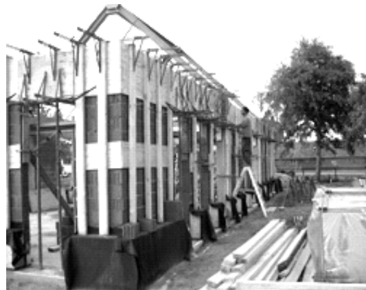
Fig 2. House using passive components, Deinze, architect: denc!-studio. The house is built as a shell with a total free interior. The lack of inner walls stabilising the construction calls for a rigid mix of brick, concrete and steel, around which a non load bearing construction out of TJI beams supports the mineral wool insulation.
