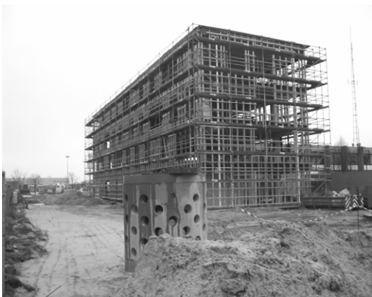
Fig 3. Certified passive office building, Ghent, architect: evr-architecten. This office building uses a traditional concrete floor slab construction, providing the necessary thermal inertia. The façade around it is a highly insulated timber frame construction, built on site.
