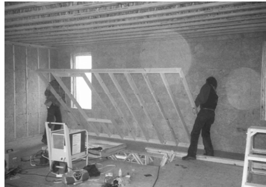
Fig 1. Certified passive house, Heusden-Destelbergen, architect: denc!-studio. The façades are constructed out of two standard timber frame constructions with a continuous layer of mineral wool insulation in between
