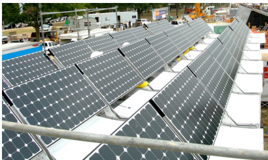
Fig. 2. PV Panels and Shade Screens, Georgia Tech Solar Decathlon House, 2007
