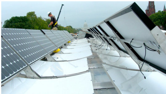
Fig. 4. Adjustable PV Panels, Georgia Tech Solar Decathlon House, 2007
