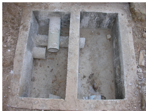
Fig. 7. Zero Discharged sewage system of the project
