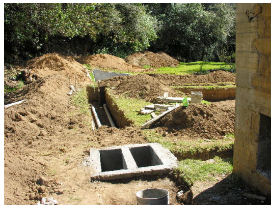
Fig. 6. View of rainwater storage and sewage systems
