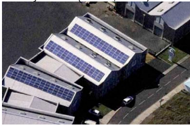
Figure 11 – Photovoltaic system with public network connection, 32 kW – Réunion Island, France.
