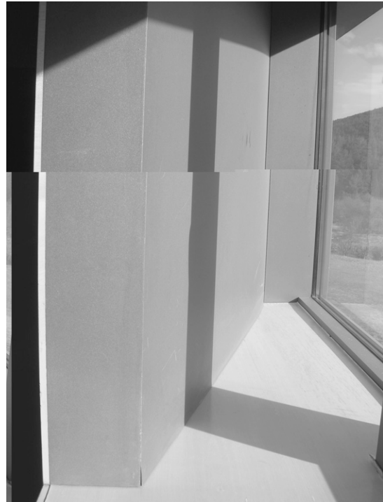
Figure 7. Absorption panel on the south-oriented façade.
