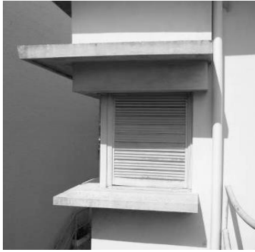
Fig 3. Solar protection and venetian blinds [9]
