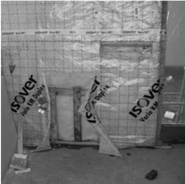
Fig 3. Phase 1 Newcastle, Problems with Airtight Membrane
