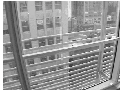
Fig 8. Spacing of the CRF in the lower portion of the office window.
