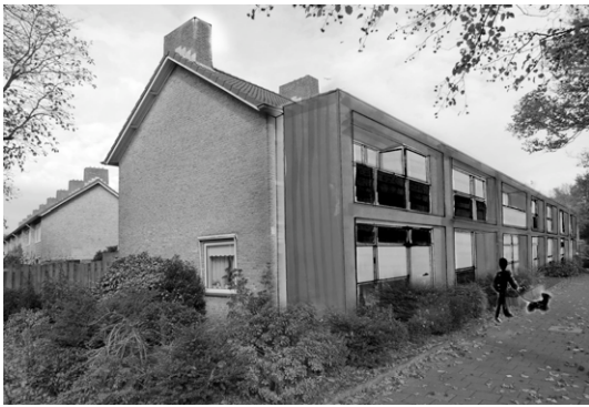
Fig 3. SmartRenovation in the front yard. The 3D connector separates the old and the new part.
