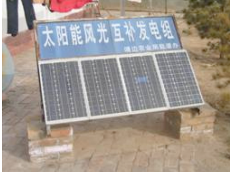
Fig 6 PV system providing electricity for night lighting and TV operation (picture taken by YAO Jiali in the Erderjing Village, Shanbei region)
