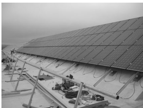
Figure 8: Photograph of bank of photovoltaic panels attached to the south facing side of the roof-light.
