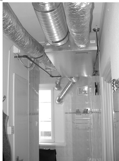
Figure 11: Installed ventilation heat recovery units under the ceiling of the hall. Now they are covered with gypsum board suspended ceiling.
