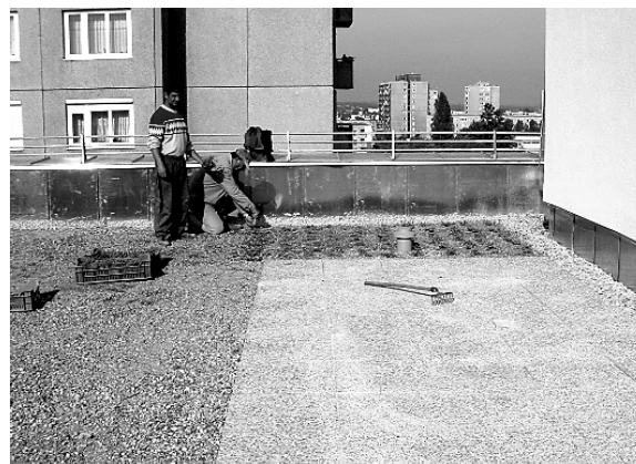
Figure 6: Planting on the green roof
