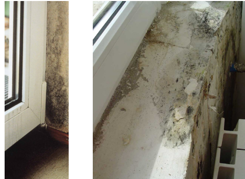
Figure 4: Airtight window produced mold on the adjacent wall
