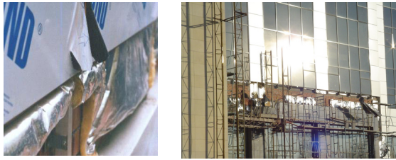
Figure 3: Aluminium vapour barrier provided on the wrong side of the thermal insulation
