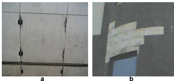
Figure 1: Deteriorated (broken or detached) marble panels: a) mechanical fixing b) „wet” fixing
