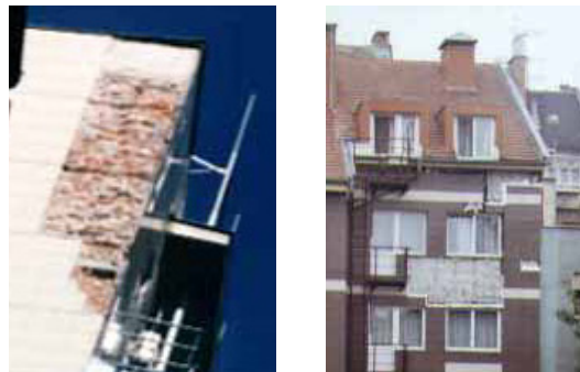
Figure 3: Detached ceramic tiles on West oriented facades.
