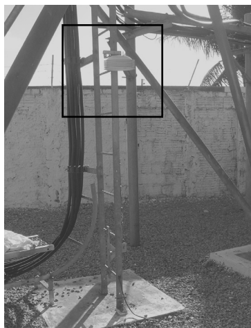
Figure 4: Installed equipment (a testator with plastic protection).
