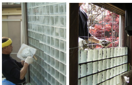
Figure 10: Laying work of glass block; finishing of joints from outside (left) and view from inside with allocating steel bars (right)
