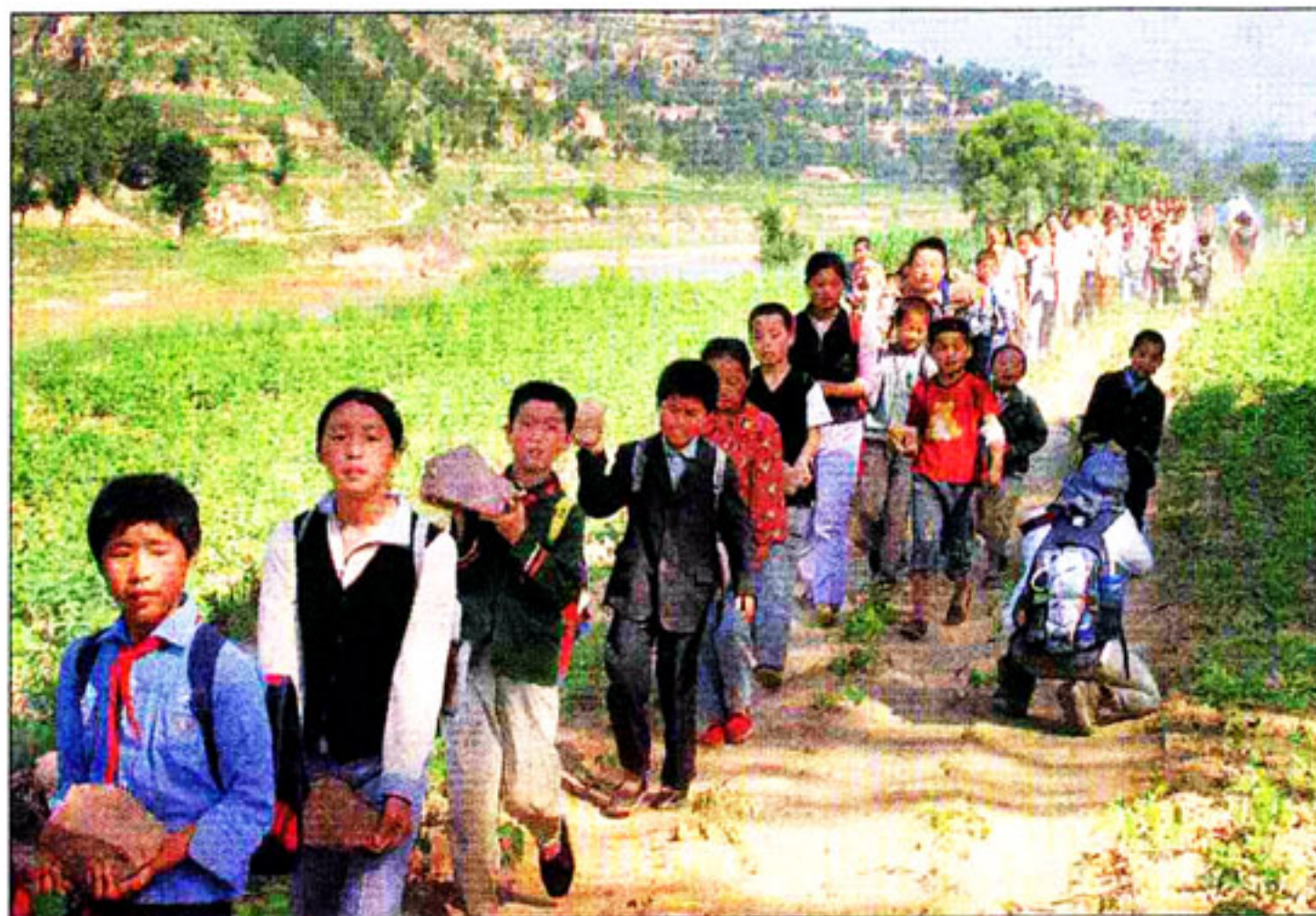
HELPING HANDS: Local children help with the construction work by carrying rocks, which are used to fill the bridge's metal frame. The journey to the school across the river is now safer.
