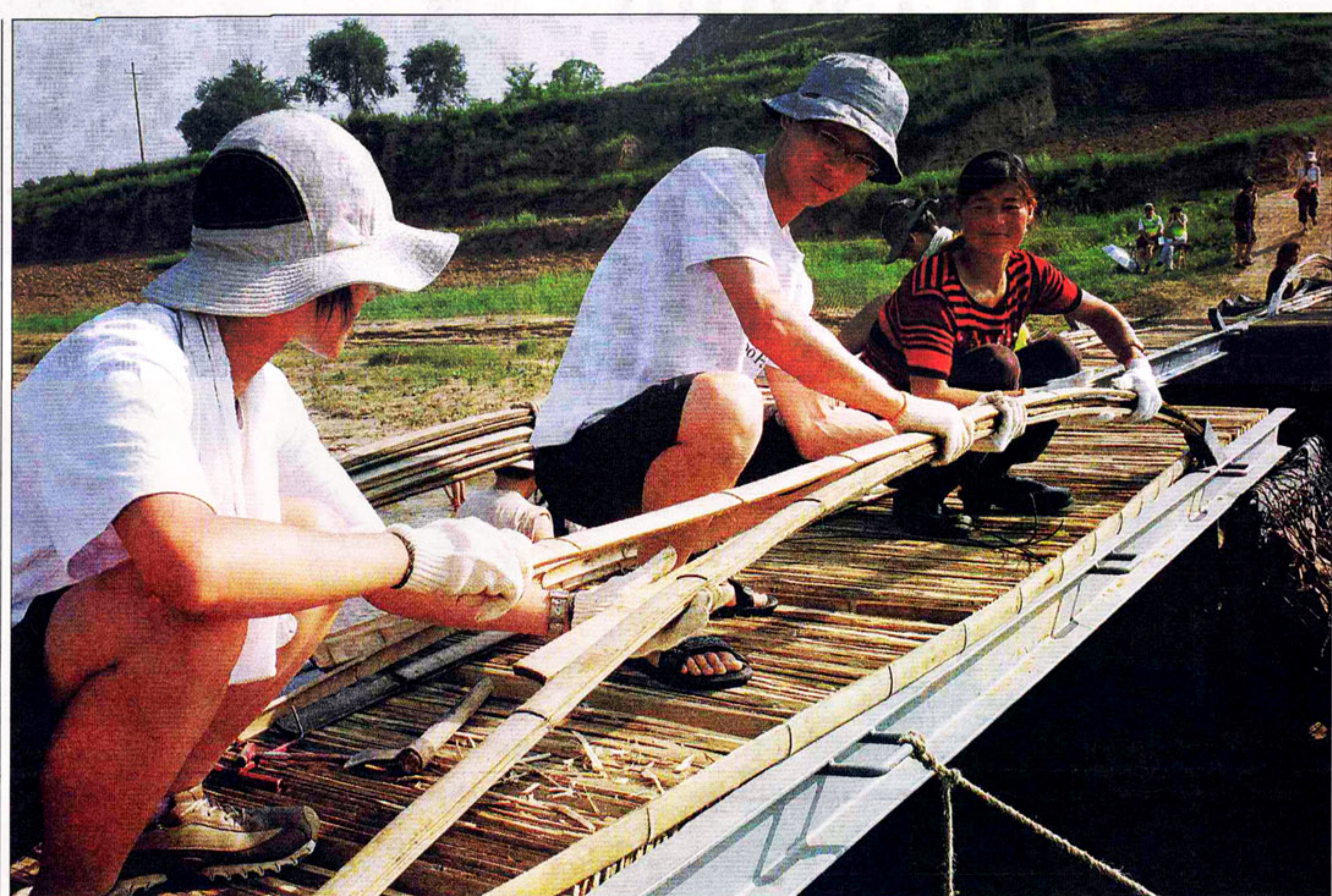
BRIDGING THE GAP: Students and villagers work together to construct the new environmentally-friendly Wu Zhi Qiao which uses mainly local natural materials. Photos: SCMP Pictures
