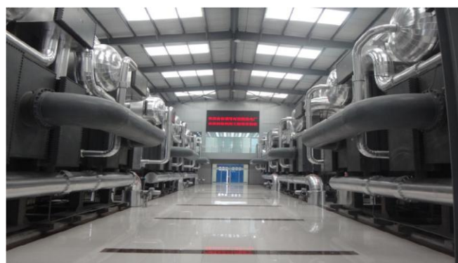
Figure 2: 5 units absorption heat pump (50 MW each)
