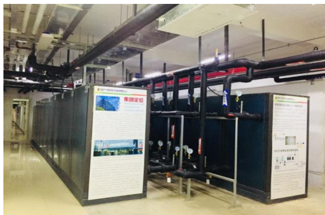
Figure 5: A 2 MWh PCM thermal storage
